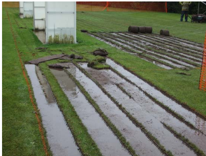
Figure 10. Waterlogged ground at Tyn-y-Wern preventing maintenance work being carried out.
