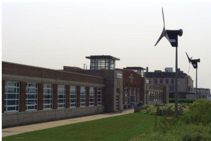
Figure 6: Example of solar PV and two 6 kW wind turbines at Blackpool Solarium
